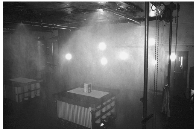
FIGURE F.3(b) Water Mist Discharge.
