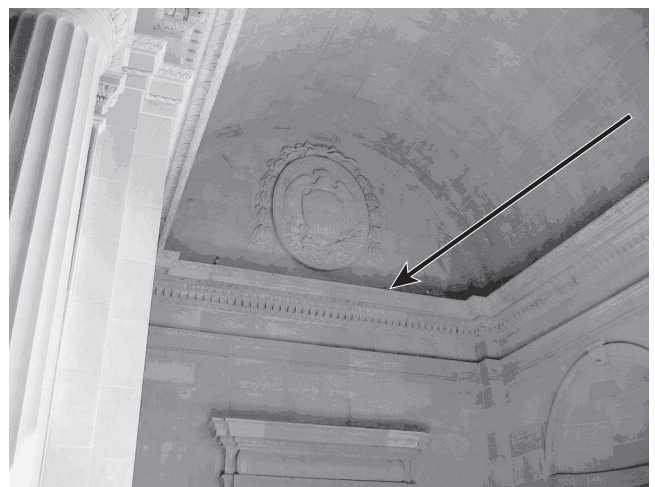
FIGURE F.3(c) Exposed Sprinkler Pipe.
