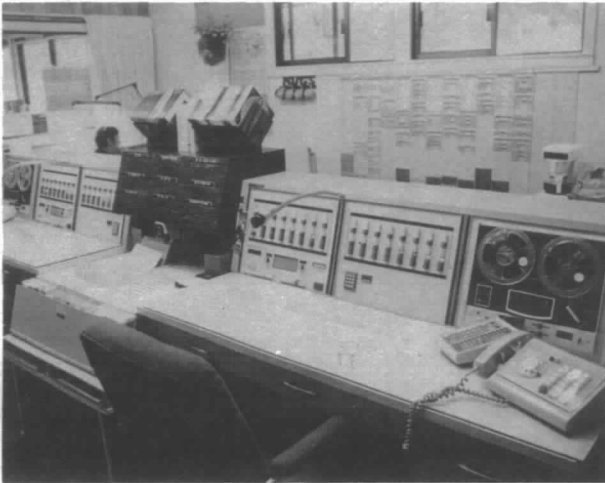
Two-position dispatch and communications console with tape recorders, response card file, and dispatch records. Note T card resource status display on back wall.
