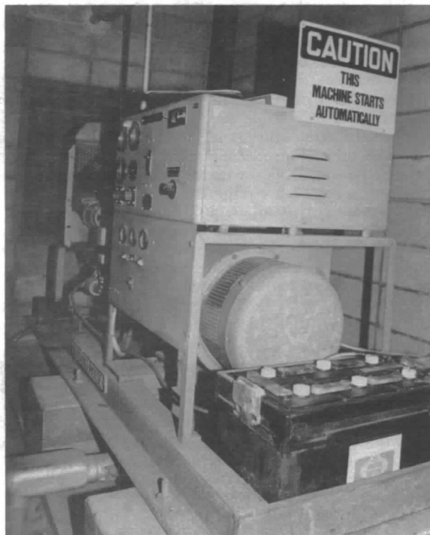
Emergency standby electric power generator.
