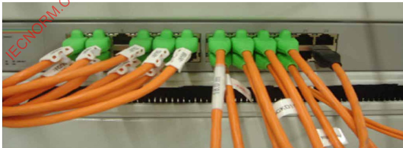
Figure 14 – Switch with copper (RJ45) ports)
