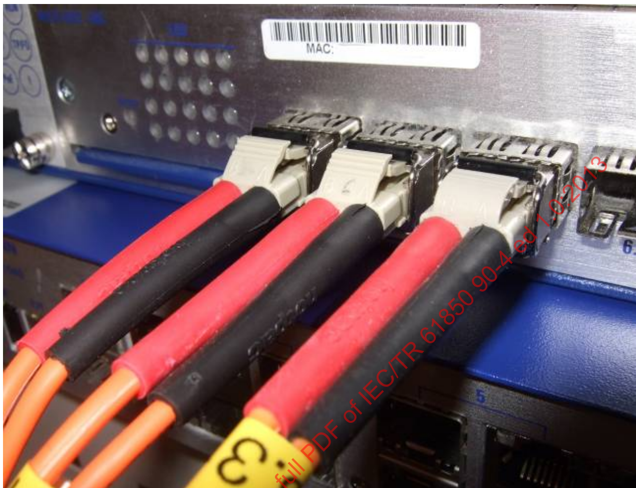
Figure 17 – Switch with optical fibres (LC connectors)
