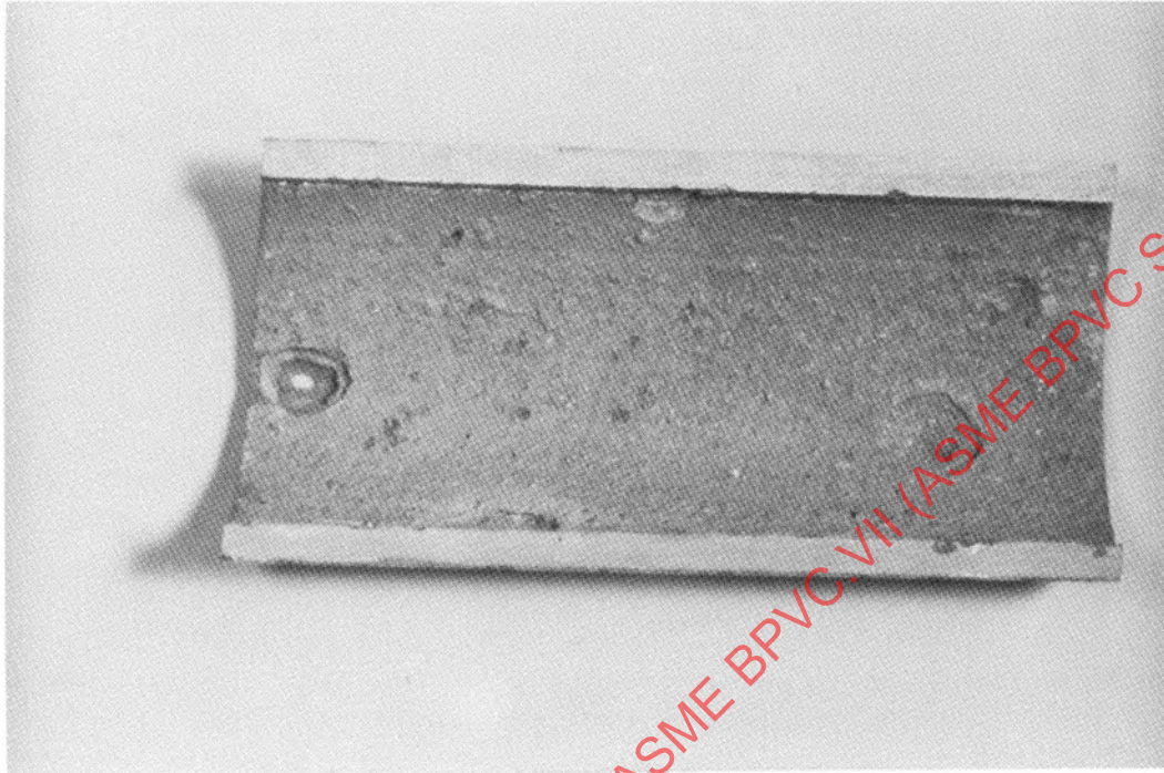
Figure 200.5.2-1 Oxygen Corrosion in an Economizer Tube
