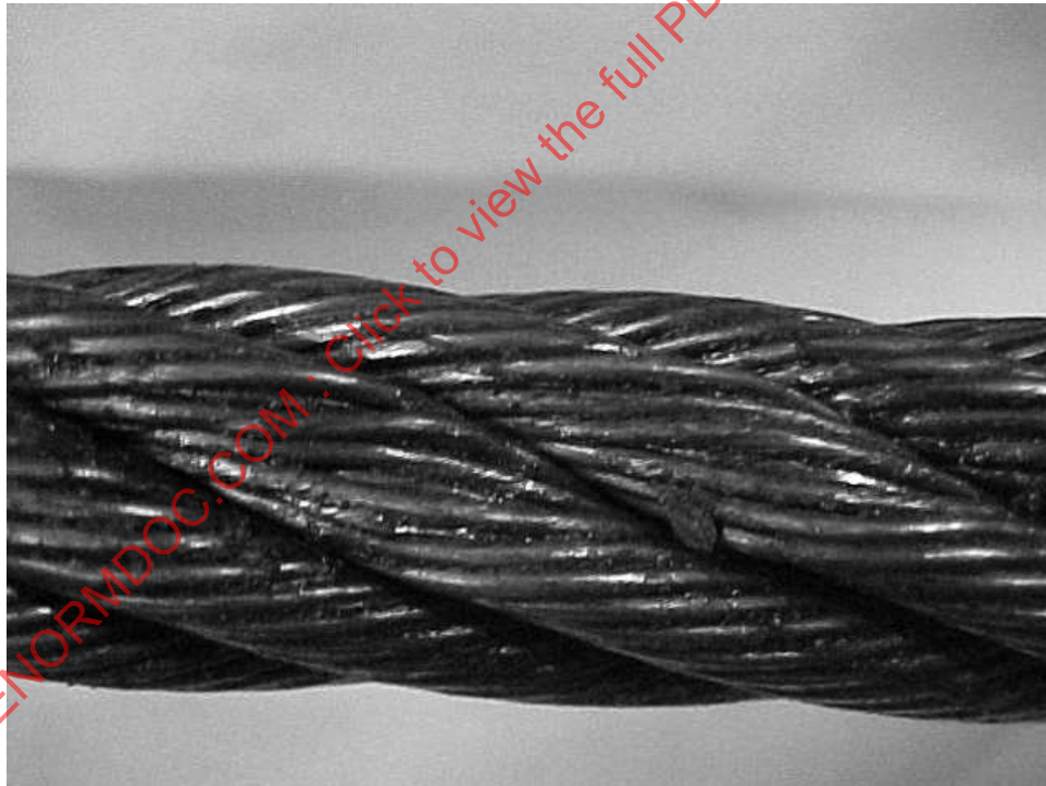
Figure 30-1.8.2-5 Distortion of Rope Structure — Crushing
